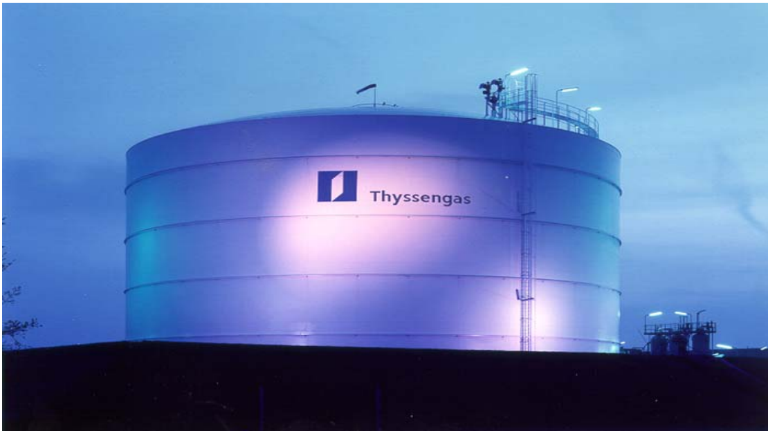
Liquid gas storage facility tank in Nievenheim
